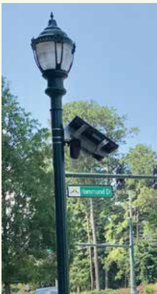
Solar & Existing Pole
