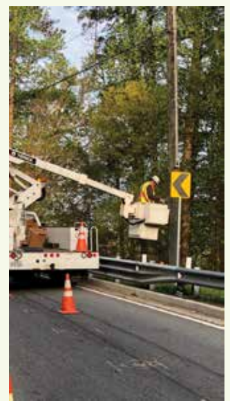
Electric & Existing Pole
